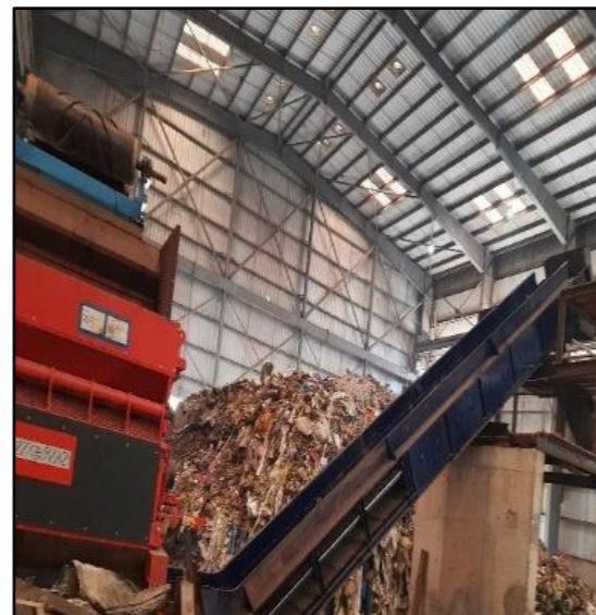
2 Weima Shredder installed
