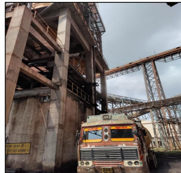
Carbon Black unloading System
