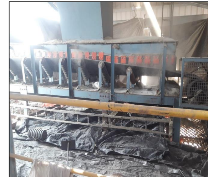
Belt conveyor installed in Line-3
