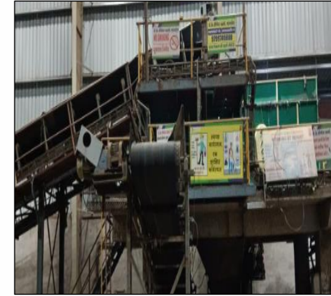
Ballistic Separator installed
